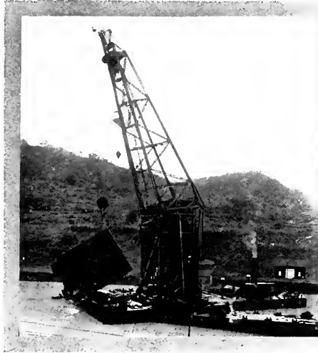
Fig. 4. Removing the wreck of the drill barge "Terredo" from the canal channel in the Cucarache section.
